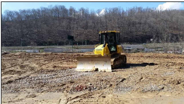
Figure 2 – Looking west across Area 3 at soils to be capped. Cap extends south to where dozer is parked.
