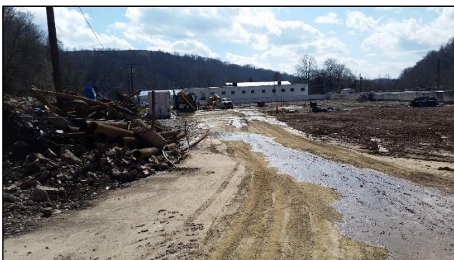
Figure 3 – Looking south at equipment wash area to be capped to prevent flow to oil/water separator.
