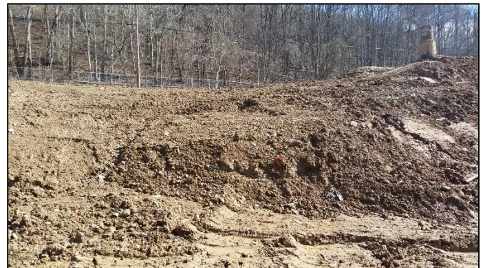
Figure 5 – Looking east up slope of Area 4. Reinforcement to extend from left to immediate foreground of photo.
