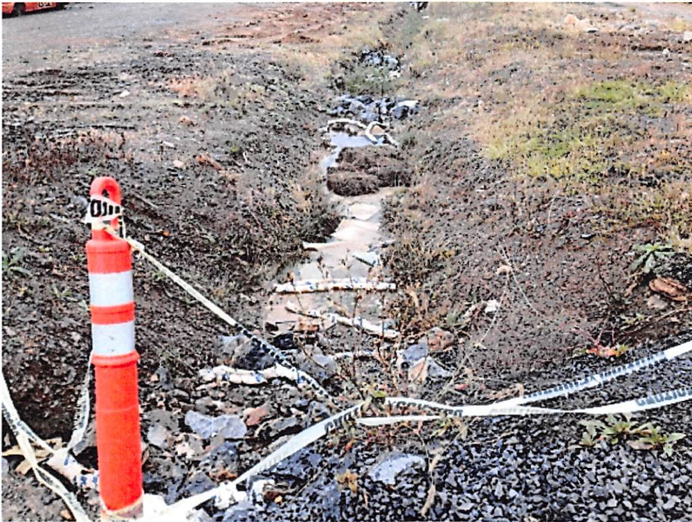
Petroleum absorbent material in a tributary feeding a wetland
