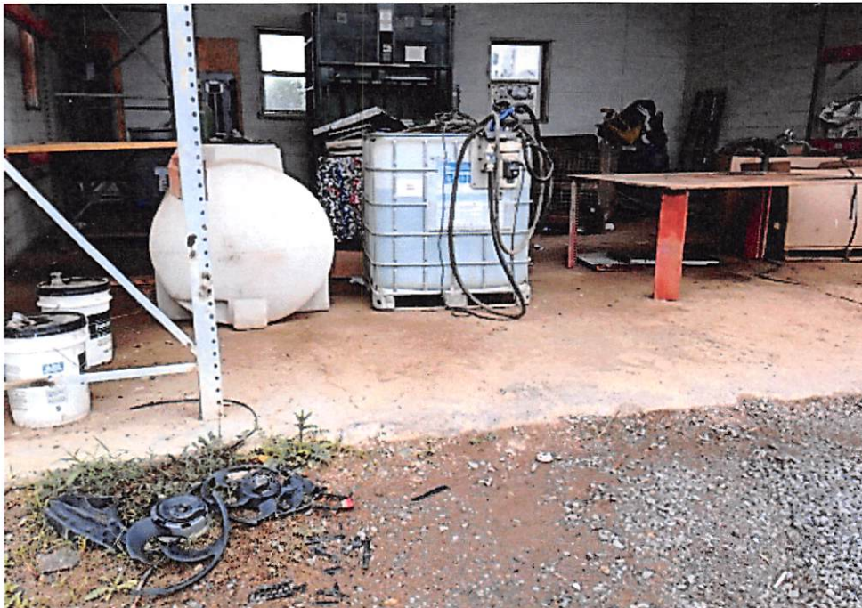
No secondary containment
