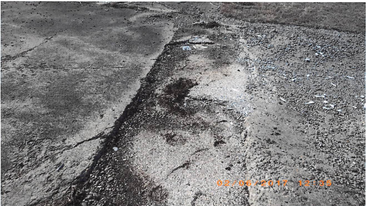
Old diesel spill -Cleanup not complete
