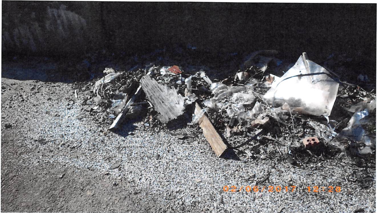
Some remaining waste
