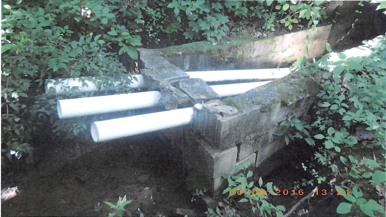
Underflow not functional at Outfall 004
