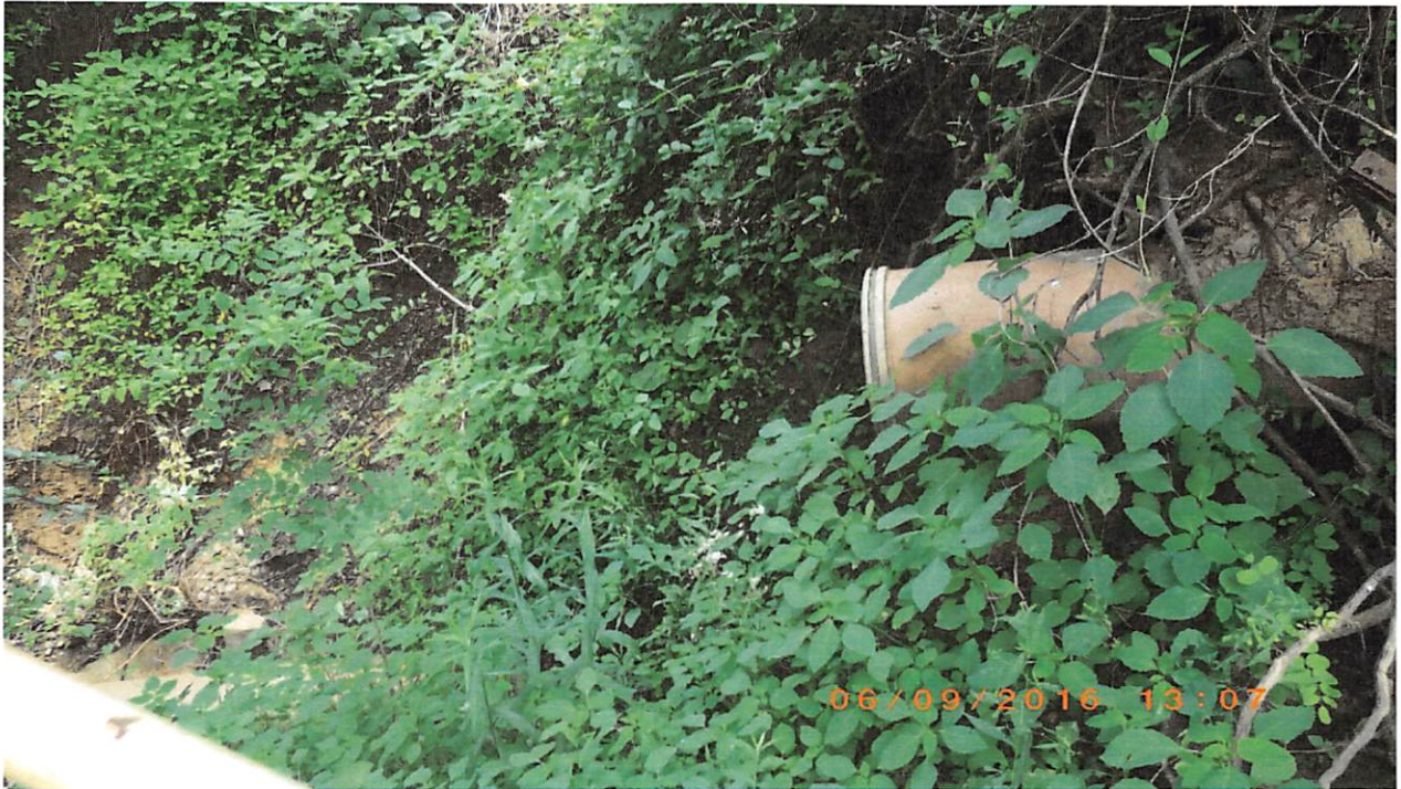
2 nd unpermitted Outfall
