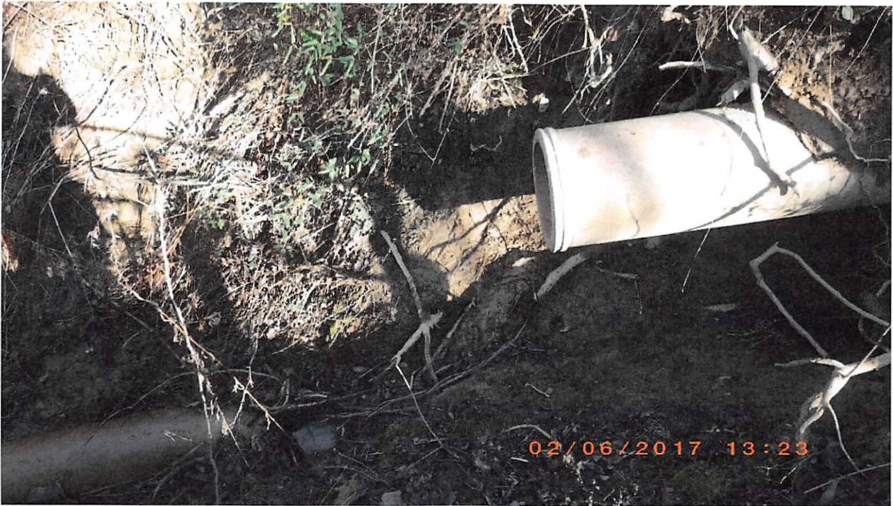
Second Unpermitted Outlet
