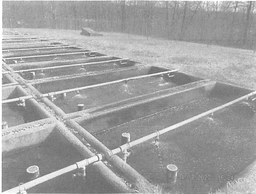
Flooded sand filters.
