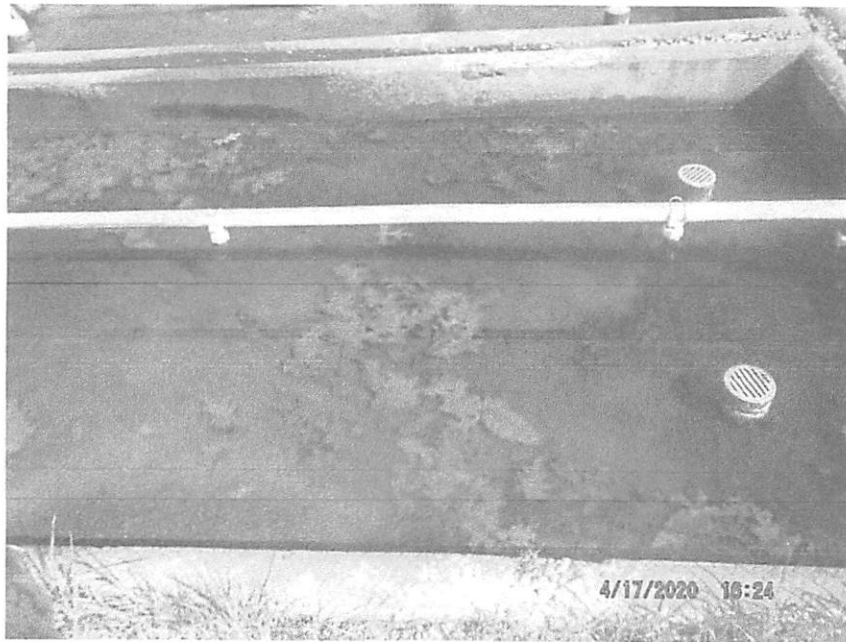
Flooded sand filter with algae and leaf buildup.
