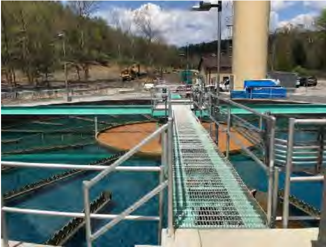
The T&T treatment facility located near Albright, WV.
