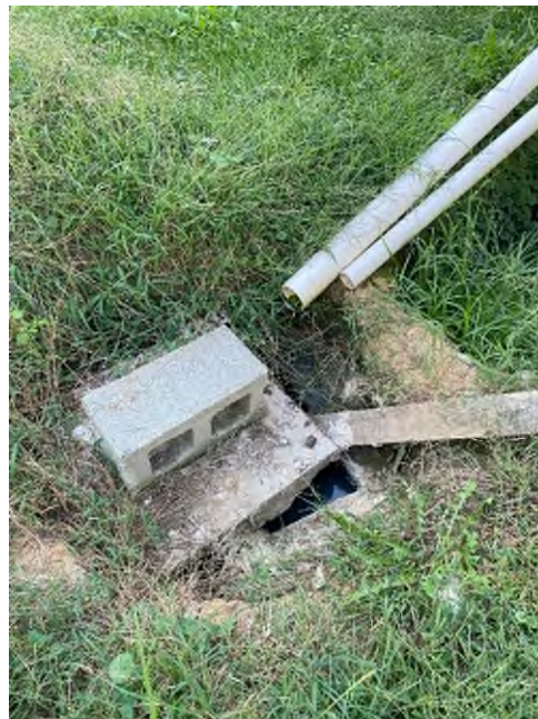
Figure 20. Failing septic tank prior to being replaced by a new system.
