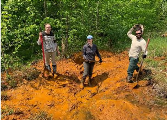
Figure 6. FODC works hard to maintain one of many acid mine drainage (AMD) treatment sites.
