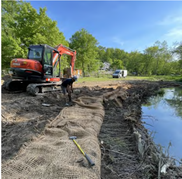
Photo left: Bank erosion on Tuscarora Creek project site in the Opequon Creek watershed, the number one priority in West Virginia's Chesapeake Bay cleanup effort.
