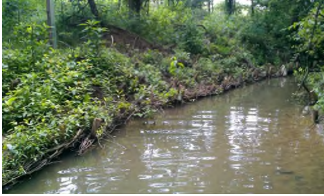
Photo left: Webber streambank stabilization project. Area was graded to a less steep bank angle and protected with brush mattress, live fascines, and live stakes. No excavation was done due to limited access, and impacts by mobilization were avoided.
