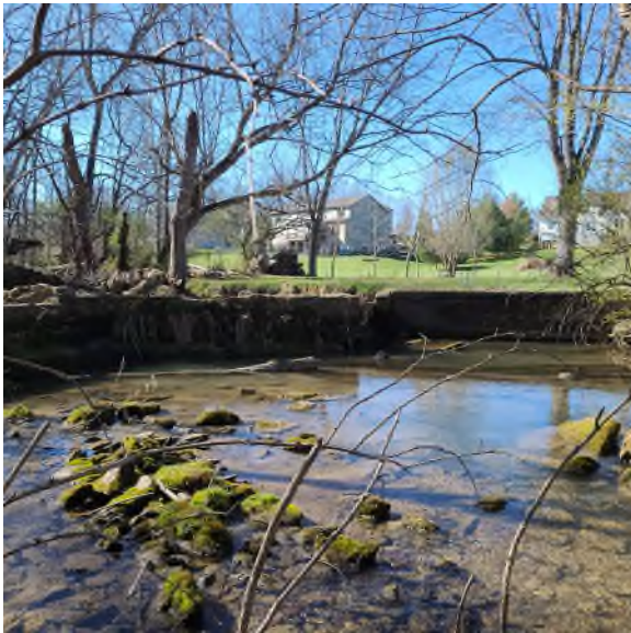
Photo left: Bank erosion on Tuscarora Creek project site in the Opequon Creek watershed, the number one priority in West Virginia's Chesapeake Bay cleanup effort.
