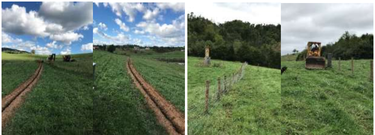
Typical view of pipeline being installed to feed an alternative watering system (left), Pasture division fence installed, and woven wire pasture division fence being stretched utilizing a bull dozer.
