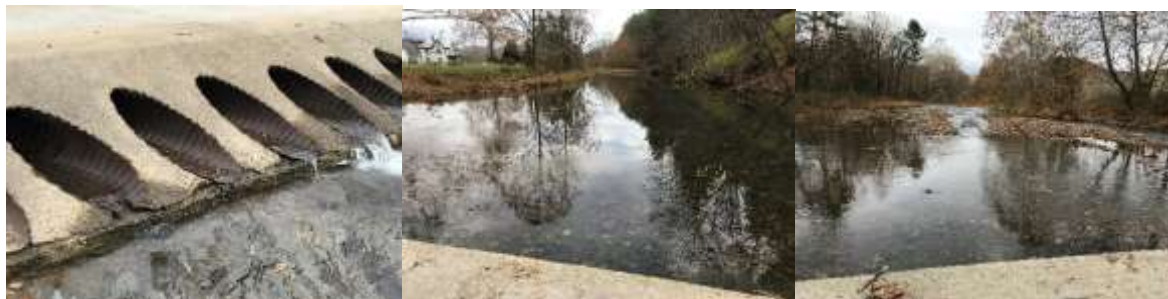
Figure 4. Left: fish passage barrier created by culvert low water crossing, Center: pool created by culvert low water crossing, Right: sediment build up created by culvert low water crossing.
