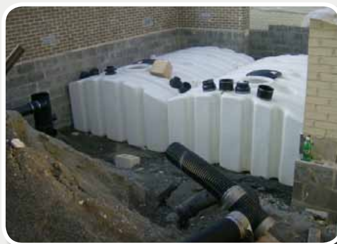
Figure RH-16. Example of two Polyethylene Cisterns (Source: Rainwater Management Solutions)
