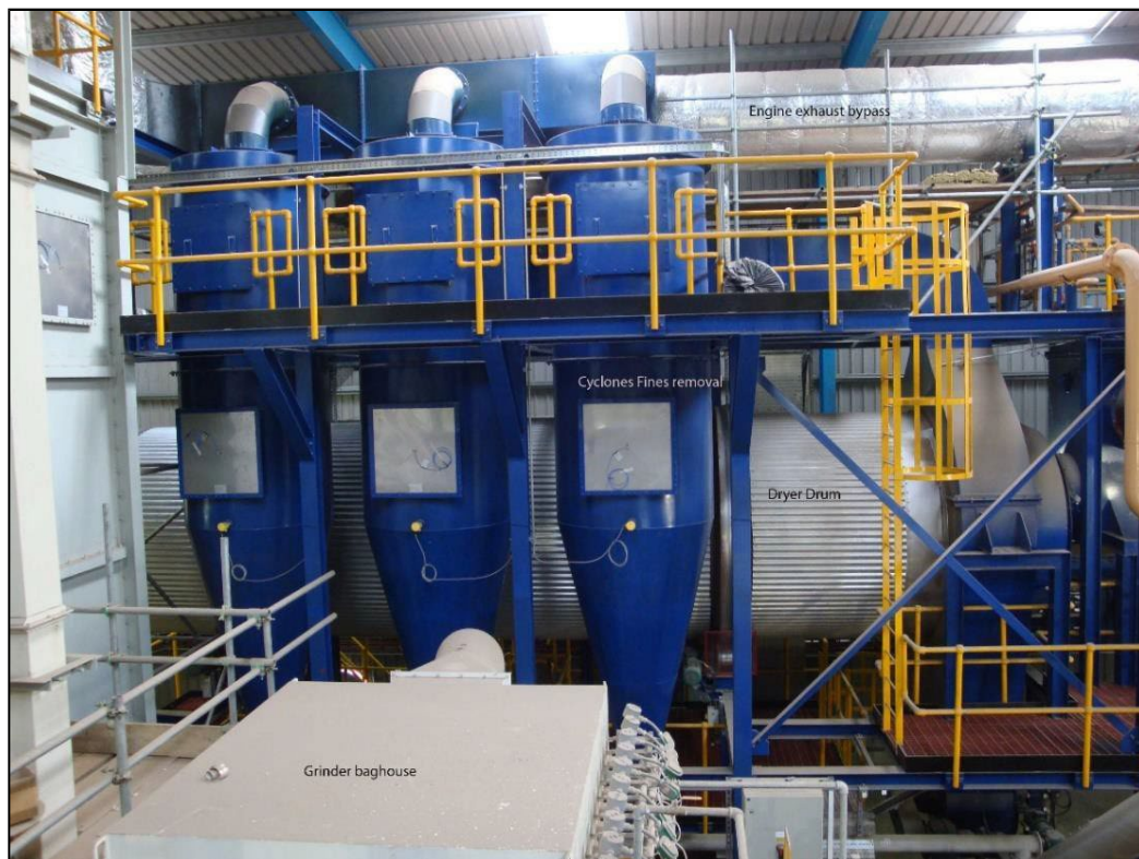
Figure 8. Photo of a typical dryer in operation from first floor level.
