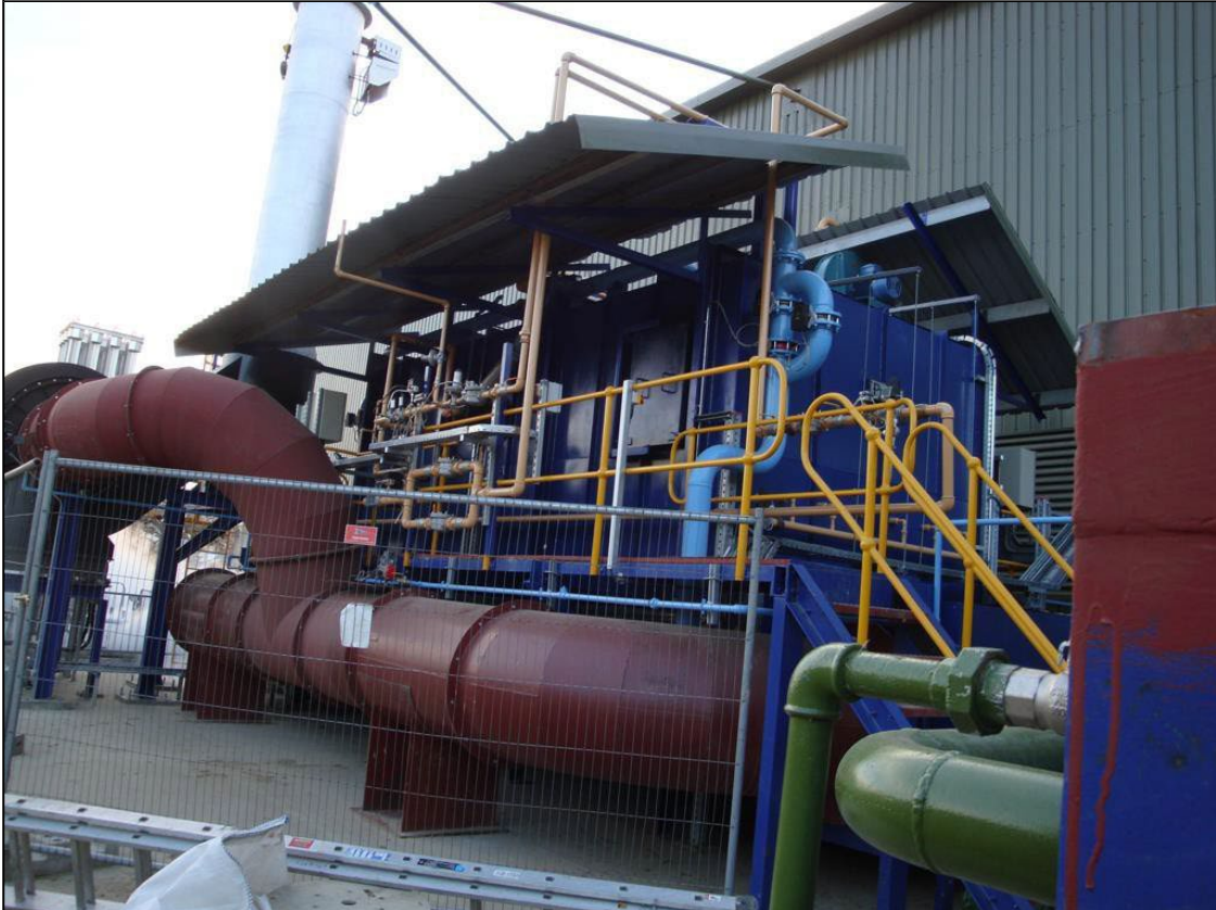
Figure 16 Photo of a typical Thermal Oxidizer in operation
