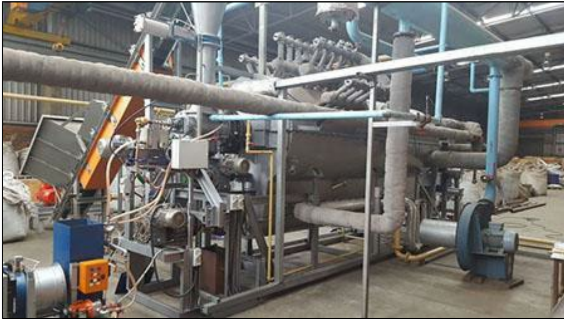
Figure 11. Photo B of typical high temperature pyrolysis unit.
