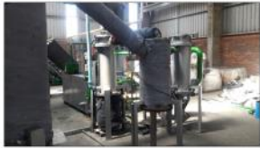
Figure 14. Photo B of a typical gas cleanup system in operation.
