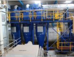
Figure 8. Photos of a typical dryer in operation from first floor level.
