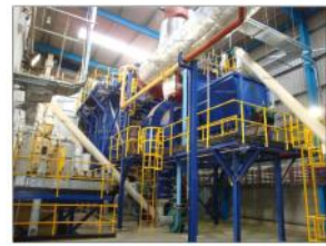
Figure 9. Photos of a typical dryer in operation from ground floor level.
