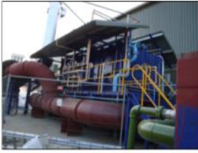
Figure 16 Photo of a typical Thermal Oxidizer in operation
