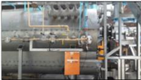
Figure 10. Photo A of typical high temperature pyrolysis unit.
