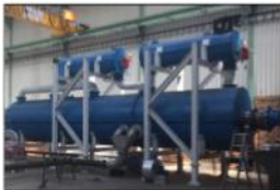
Figure 12. Photo of typical low temperature pyrolysis unit.
