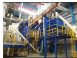
Figure 9. Photo of a typical dryer in operation from ground floor level.
