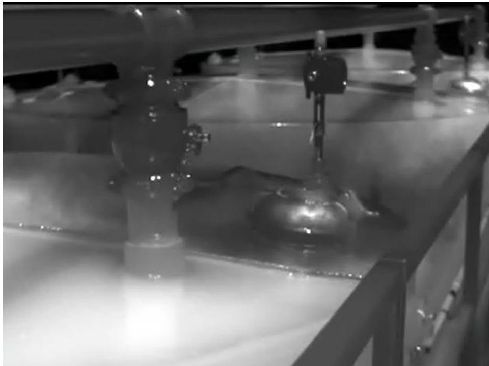
Condensate Tank Thief Hatch Vapor Leaks
