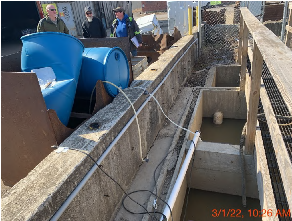
Inadequate secondary containment for Drums of PremierFloc 4240
