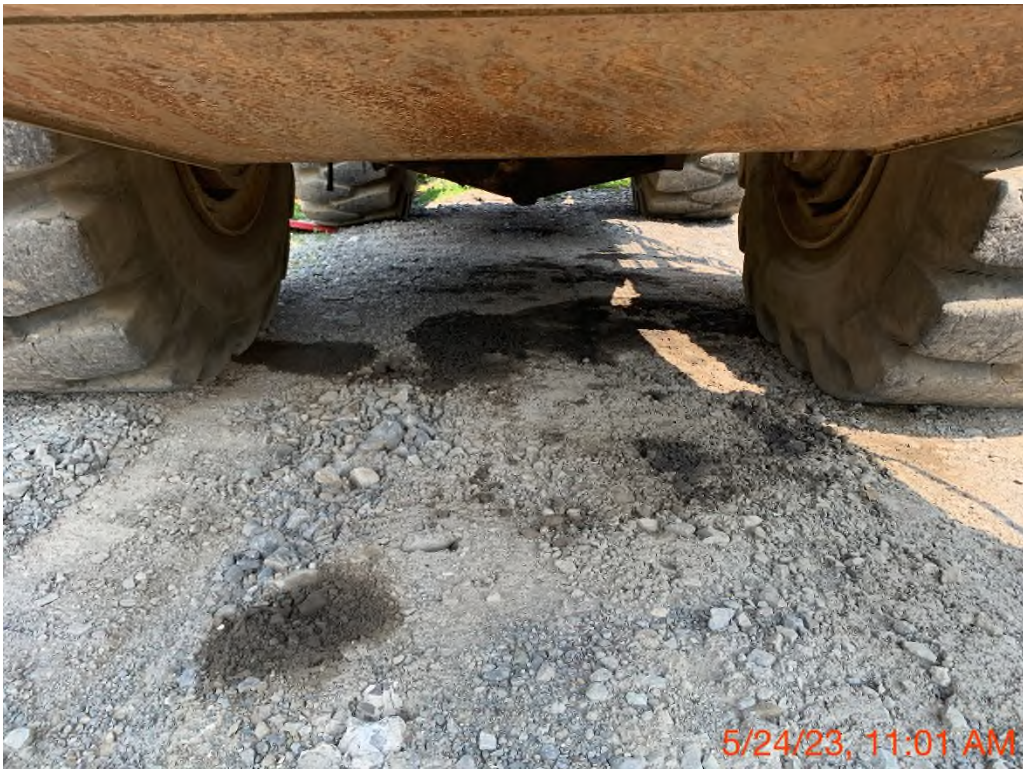
5/24/2023 There was staining on ground from equipment.
