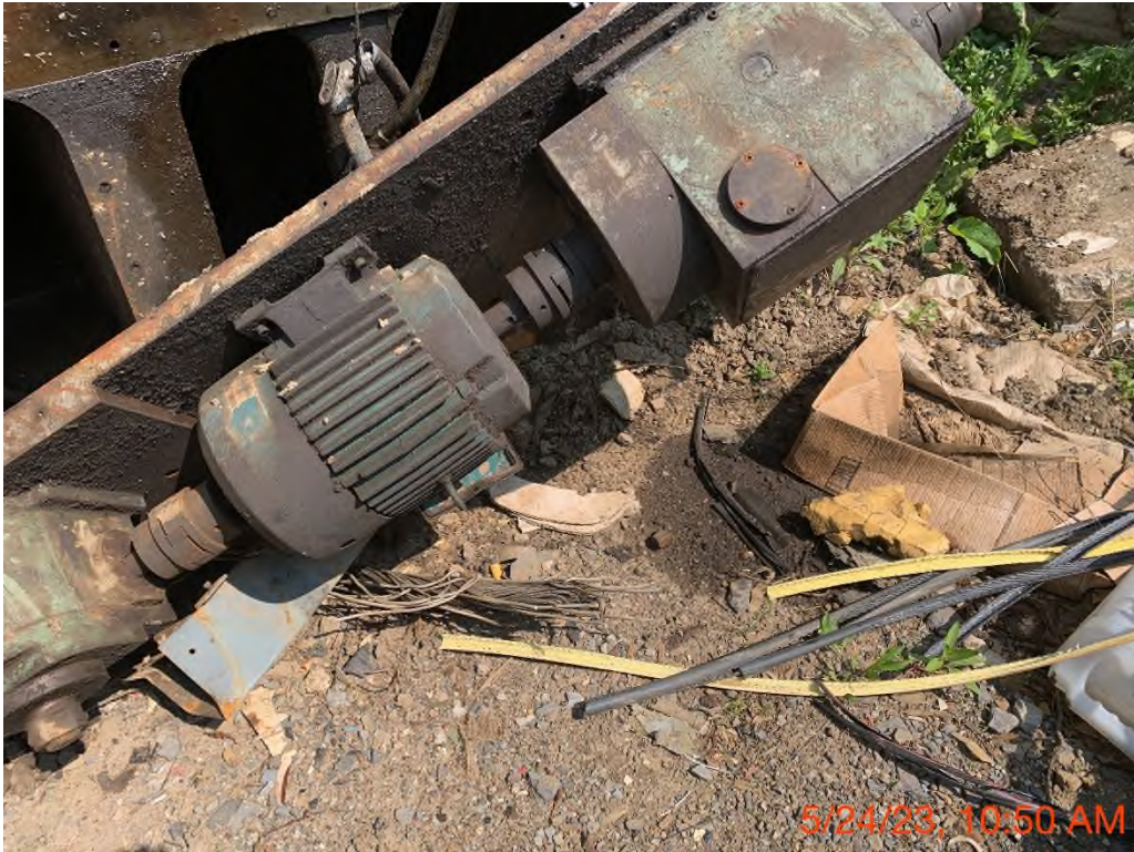
5/24/2023 There was staining on ground from equipment.
