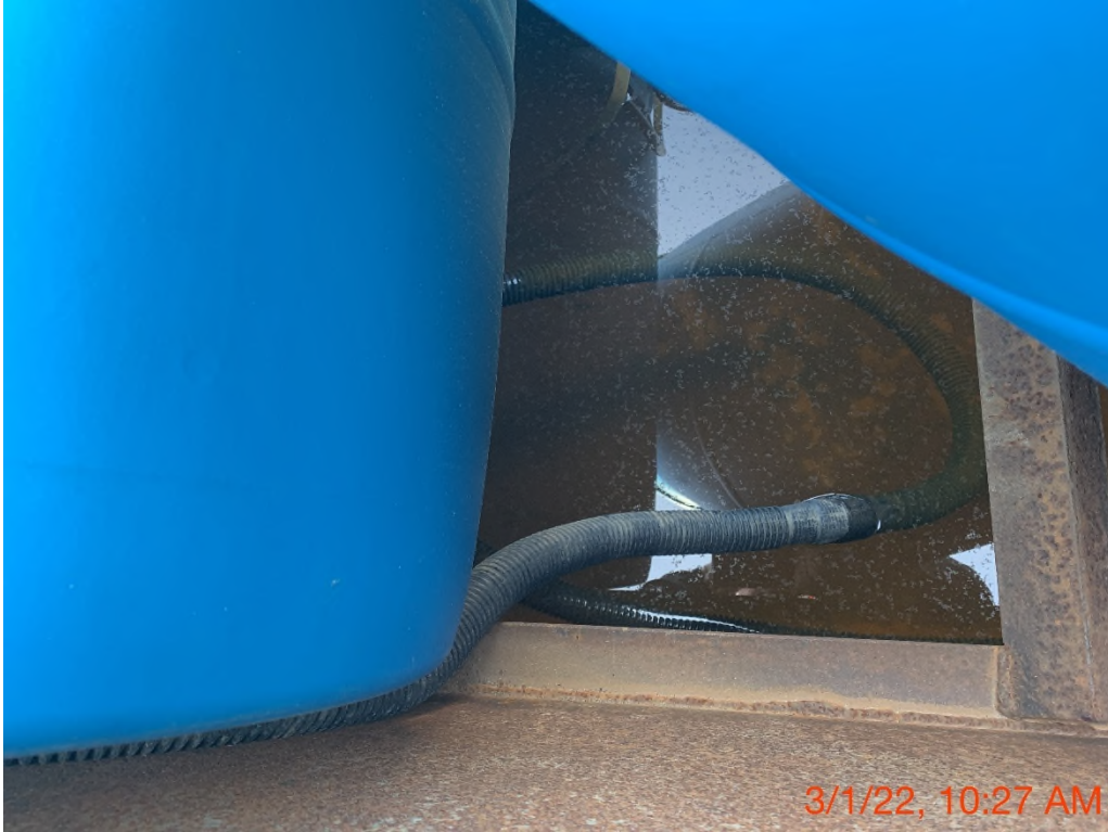
Accumulated contaminated water in secondary containment
