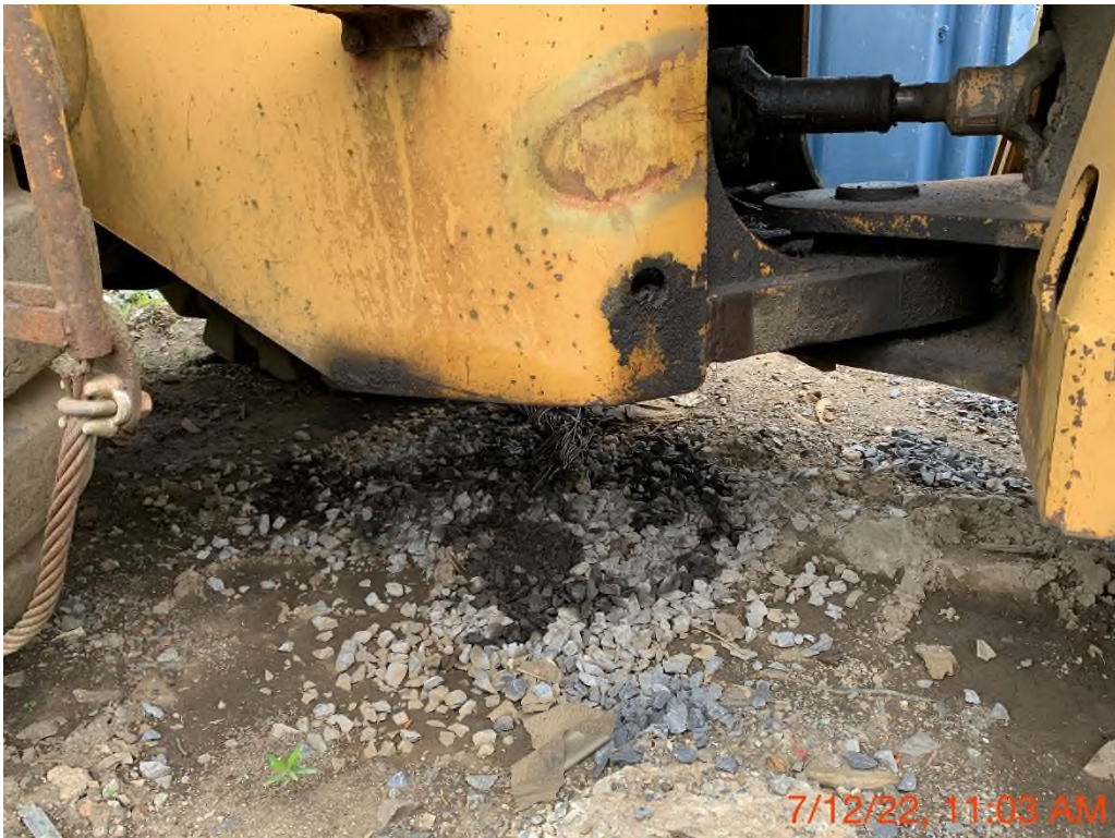
7/12/2022 Petroleum was leaking from equipment.
