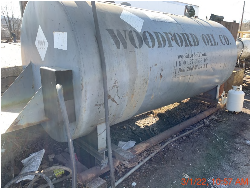
Fuel staining on the ground below the tank
