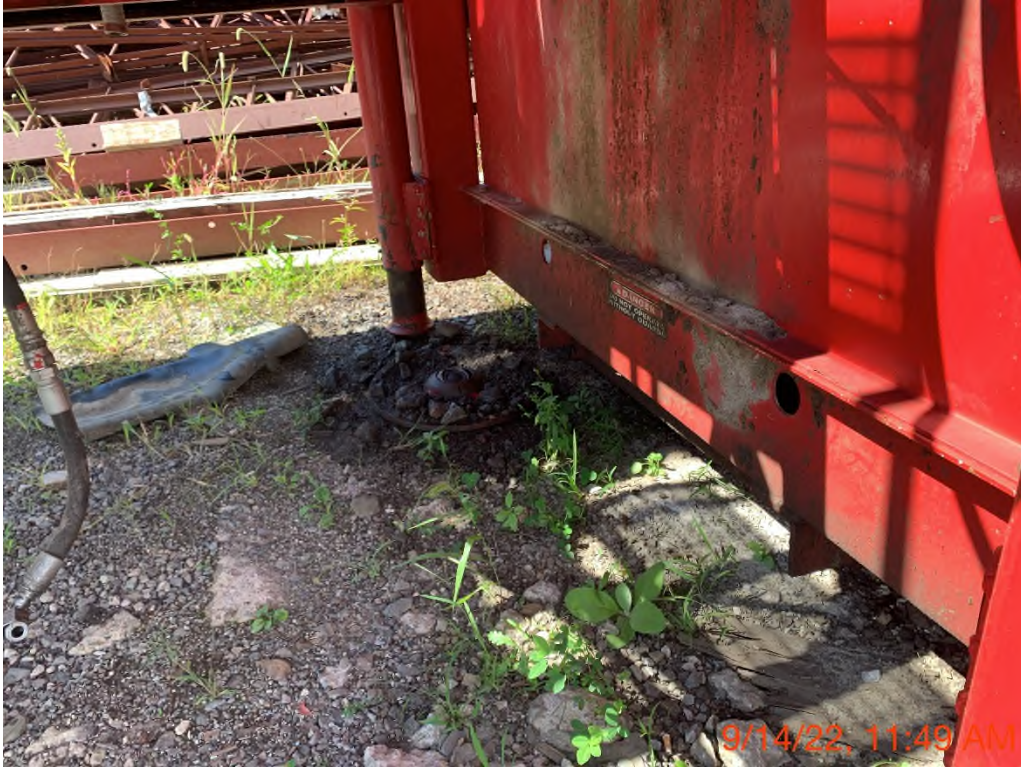
9/14/2022 There was petroleum staining on the ground.
