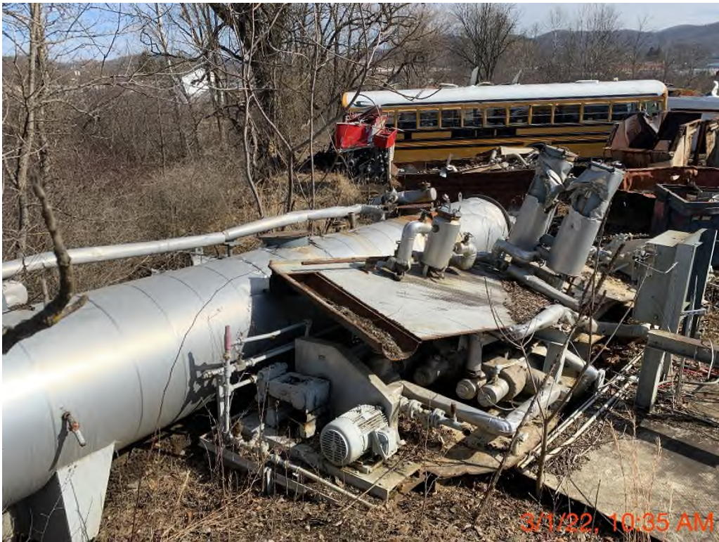
No berm installed in this area
