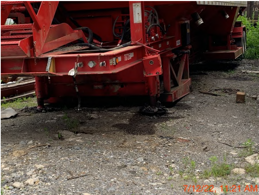
7/12/2022 Staining around hopper trailers.
