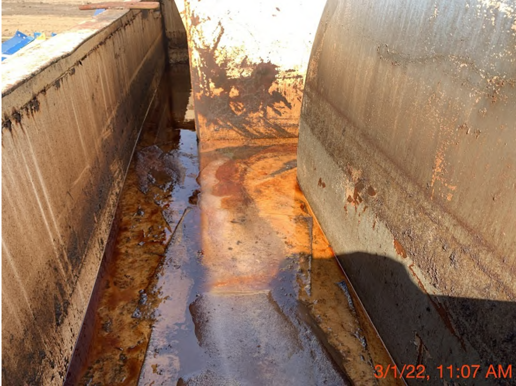
Secondary containment with petroleum contaminated water
