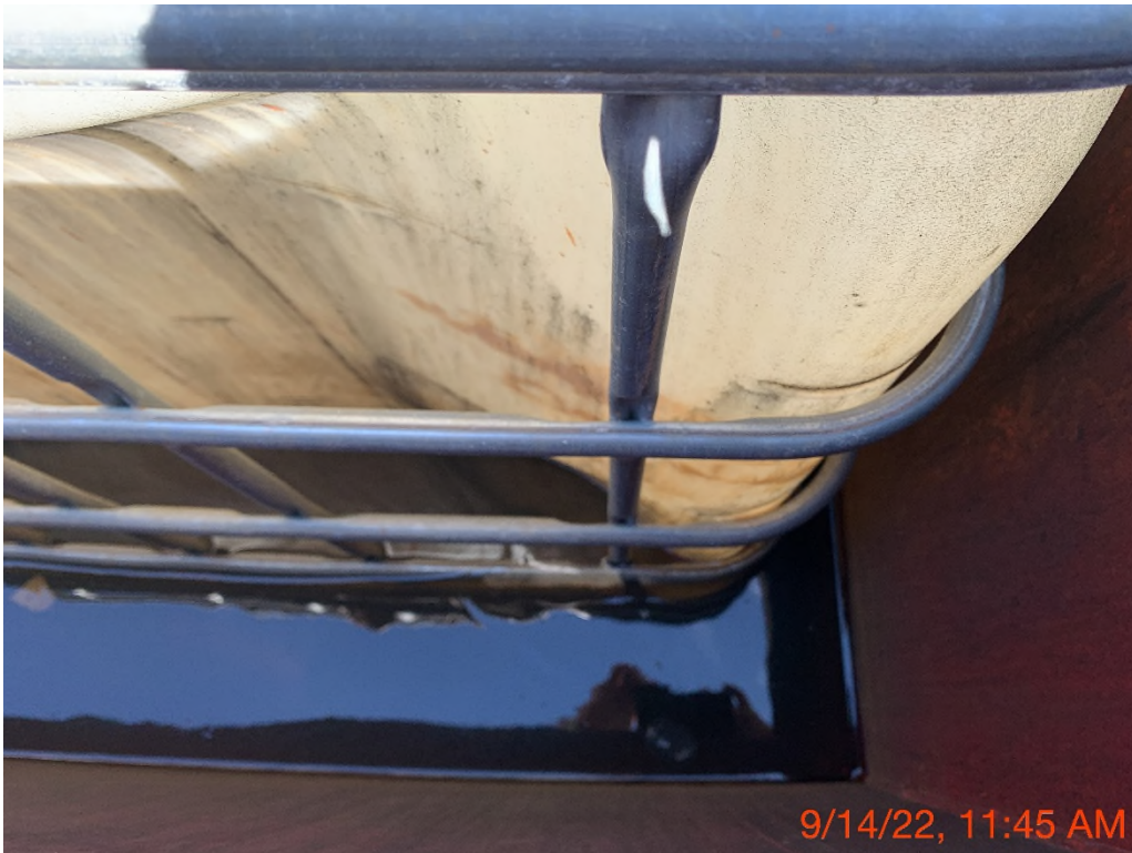
9/14/2022 Petroleum (used gas) contaminated fluids had accumulated within secondary containment.
