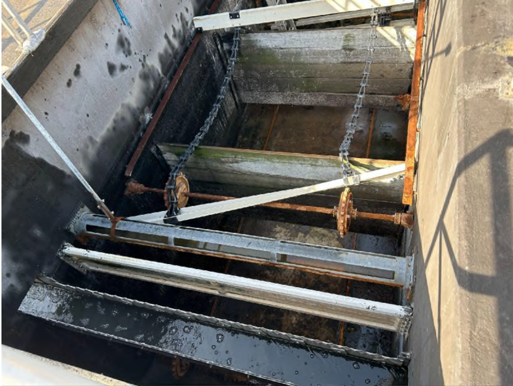
2/26/2024 IMG_3671 The secondary clarifier was out of service.
