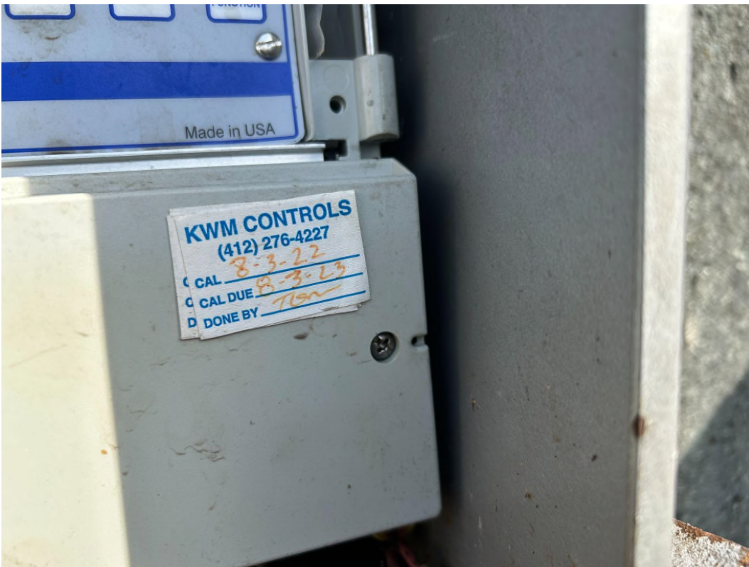
2/26/2024 IMG_3672 Expired flow meter calibration sticker
