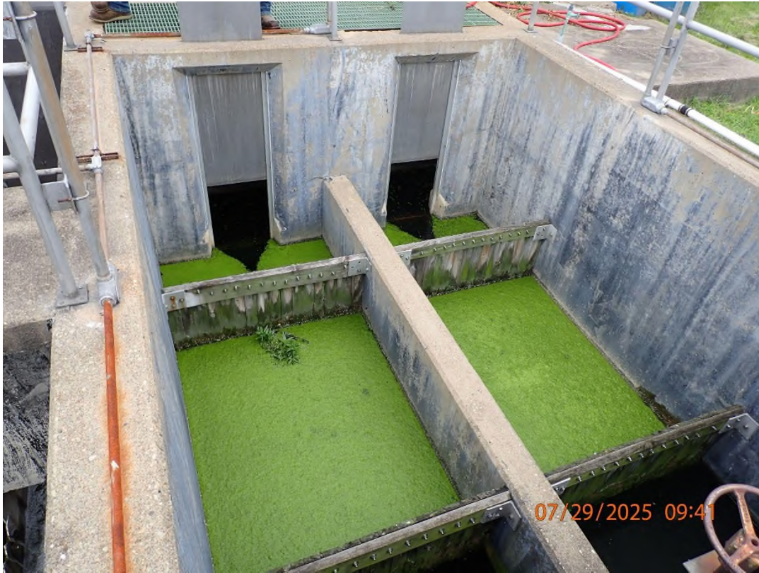
7/29/2025 - P7292020 - Chlorine Contact Chamber Covered in Duckweed
