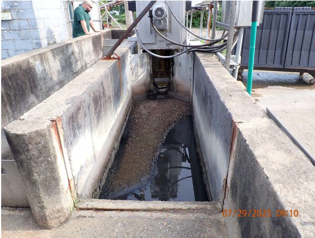
7/29/2025 - P7292007 - Mechanical Bar Screen with Solids Buildup
