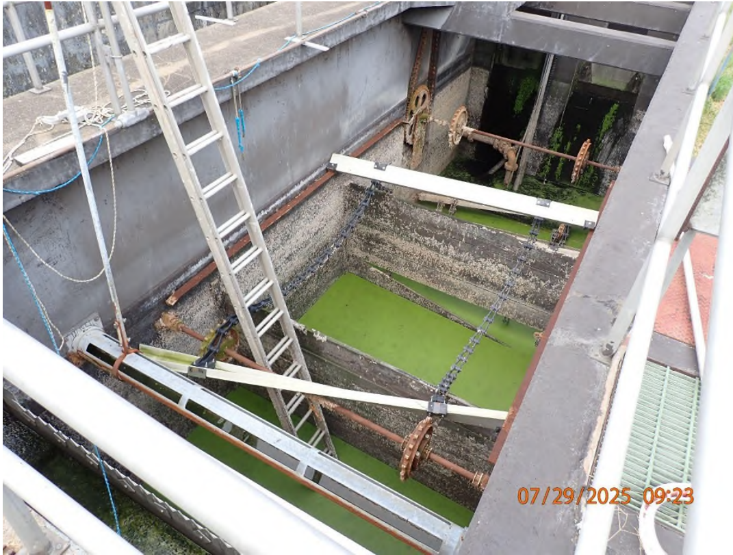
7/29/2025 - P7292011 - Broken North Clarifier Covered in Duckweed
