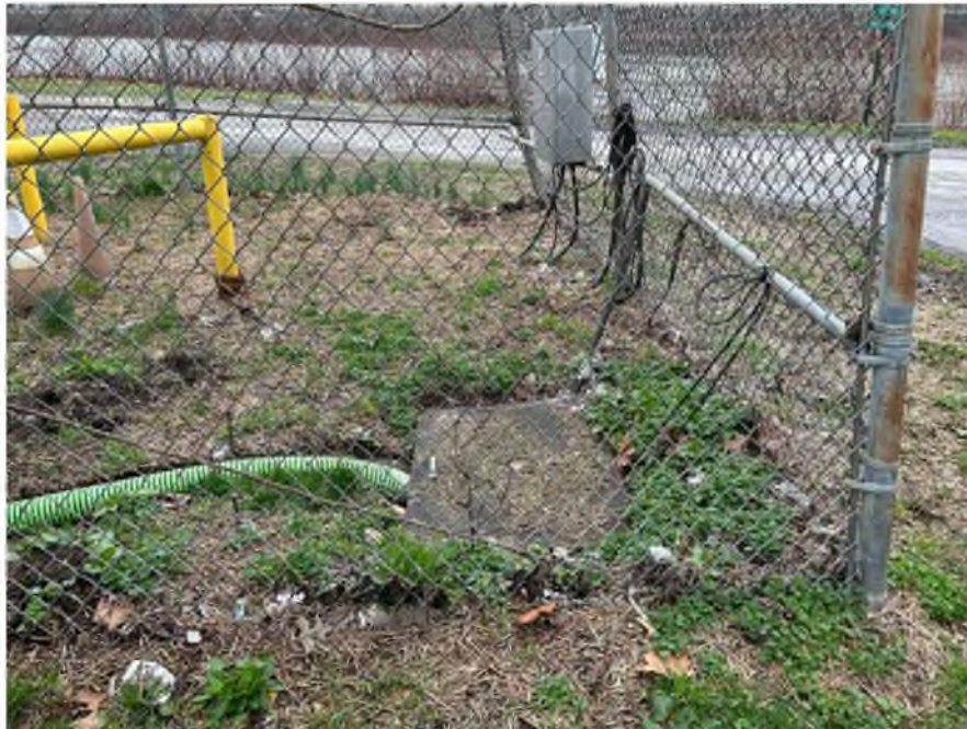
2/26/2024 IMG_3073 Pump station at C002 with evidence of overflow.
