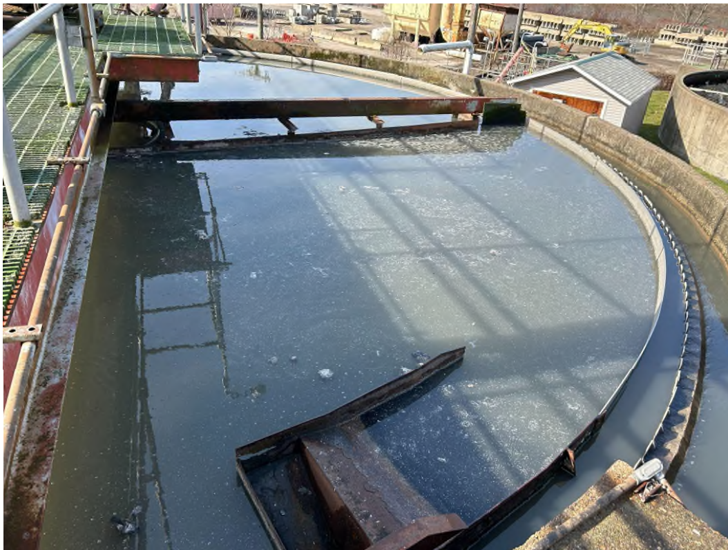
2/26/2024 IMG_3665 Modified clarigester that did not have operational rake and scum removal arms.
