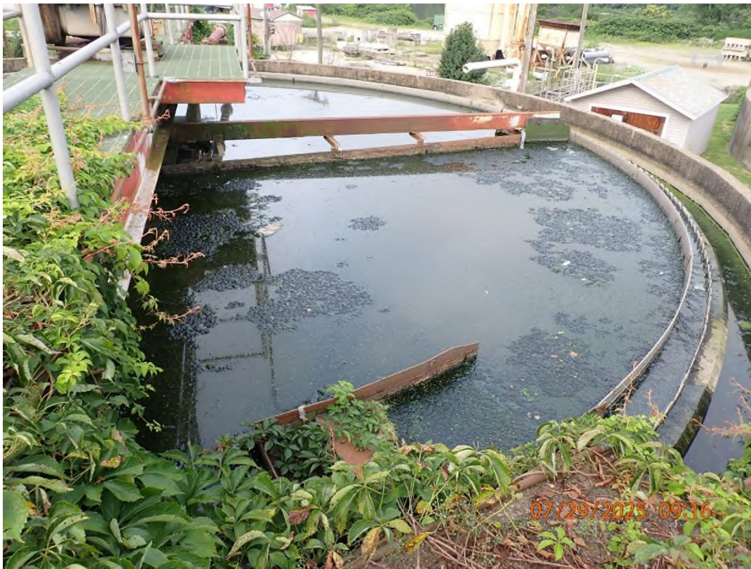
7/29/2025 - P7292008 - Clarigester with Excess Solids and Vegetation
