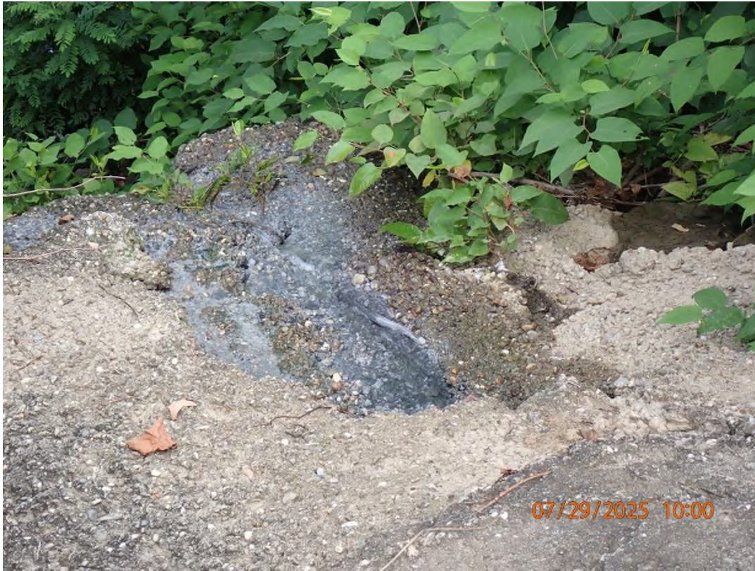
7/29/2025 - P7292027 - Outlet C002 discharging in Dry Weather
