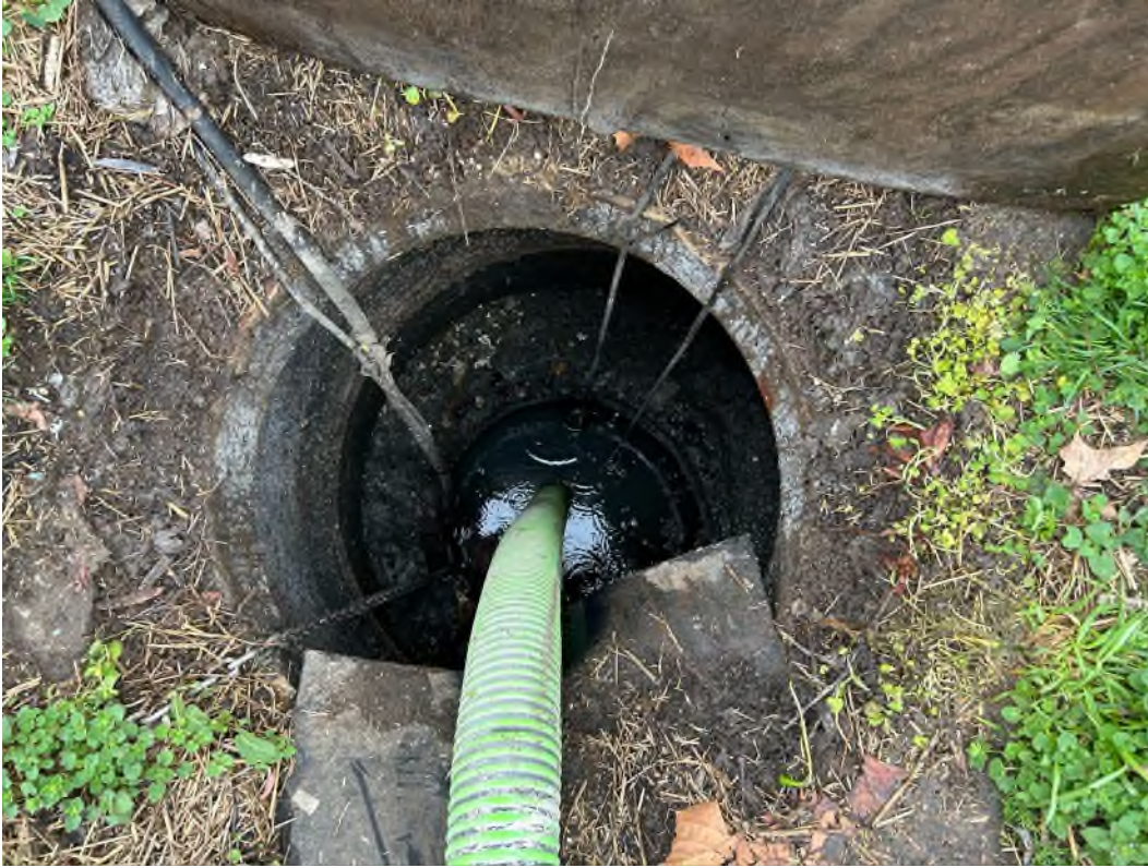
2/26/2024 IMG_3704 Well at C002 pump station had a submersible pump.
