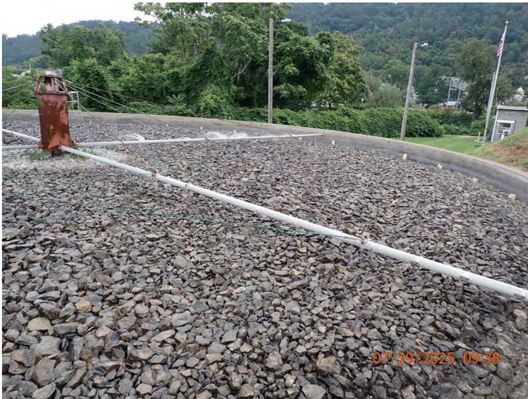
7/29/2025 - P7292017 – Only Two Arms of the Trickling Filter Operational
