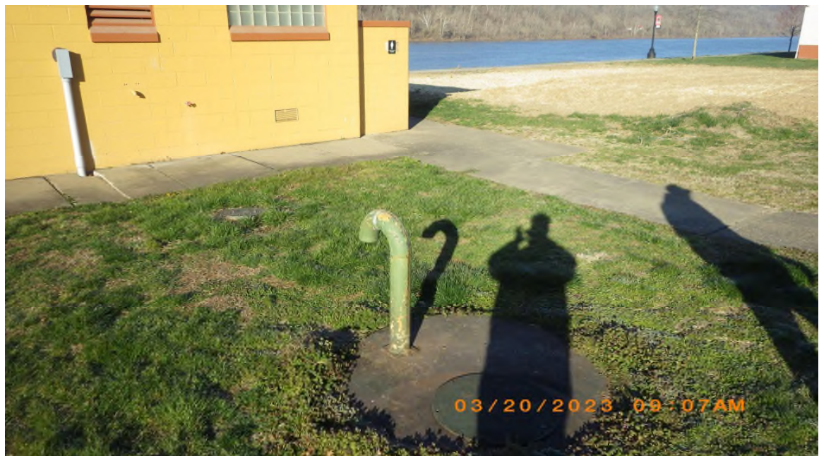
Park Lift Station
