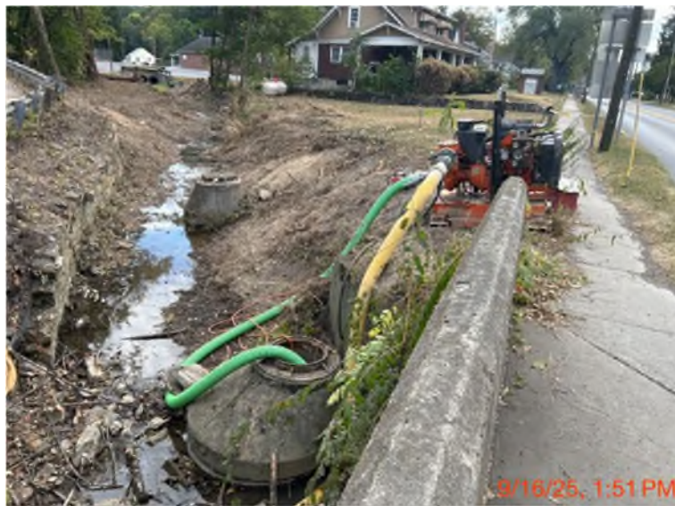
Sewer pump-around with no erosion and sediment controls in place.
