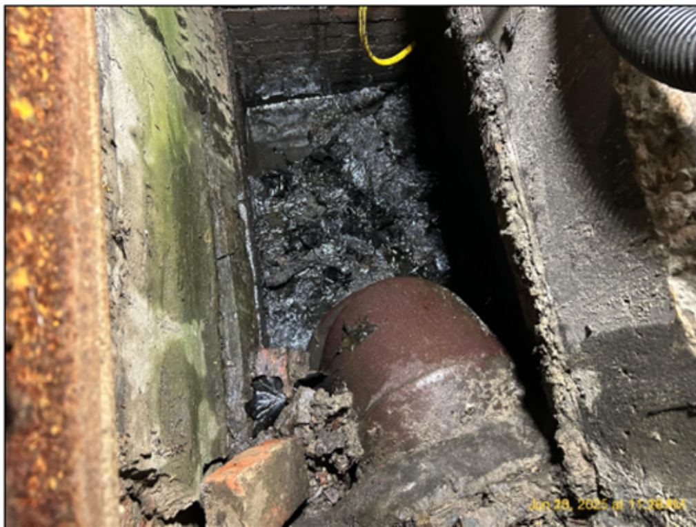
Photo 5: The vault, after cleanout by Enviroserve.
