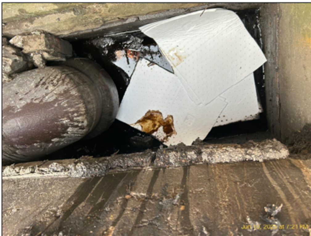
Photo 4: Oil/Petroleum absorbent pads had been added to the vault.
