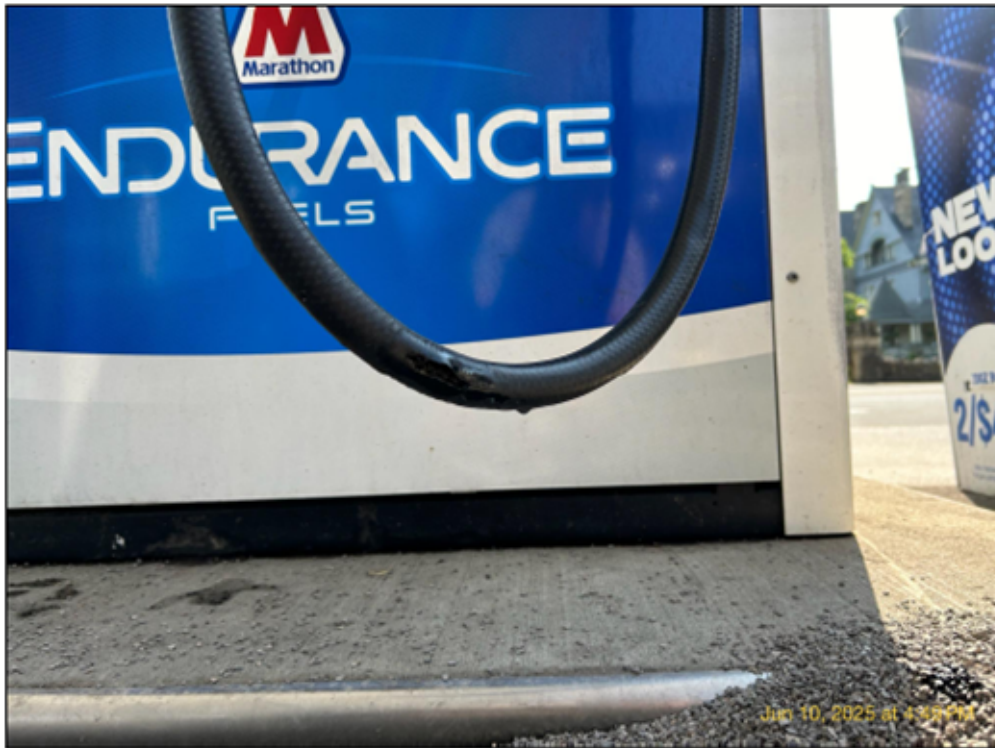
Photo 1: A leaking hose on the gasoline dispenser.
