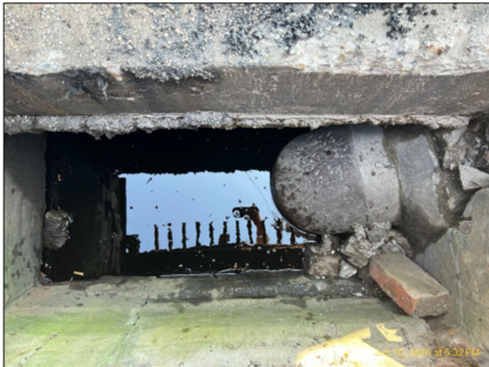
Photo 2: The initial vault status upon arrival.
