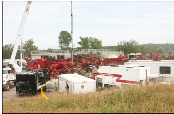
Marcellus Shale natural gas drilling operations, like the one pictured above in Upshur County, are much larger than the conventional gas well sites most people are used to.
