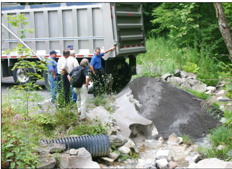
In addition to the doser sites on Abram Creek, limestone sand will be periodically dumped at three other locations. Fairfax Materials Inc., is providing and transporting materials for one year to the three limestone sites. The Abram Creek project was designed and engineered in house by staff from the Office of Abandoned Mine Lands and Reclamation.
