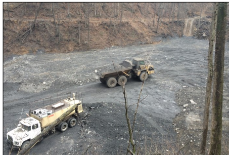
Once cooled, the material is hauled up the hollow and then covered. The valley will eventually have a grouted rip-rap channel for surface water.
