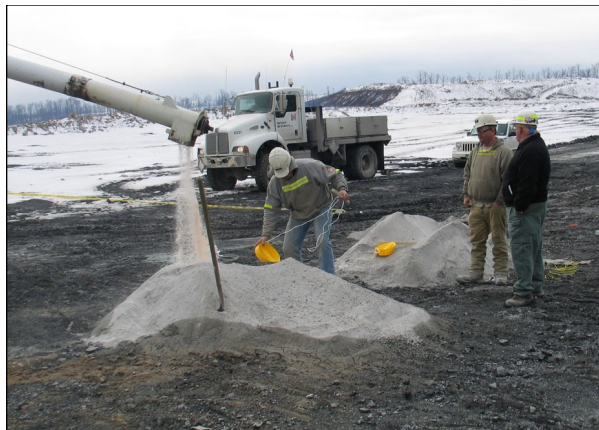
As Gary Peterson looks on, blasters at the Black Castle surface mine pour the explosive ANFO (ammonium nitrate/fuel oil) into blast holes for an upcoming shot.
