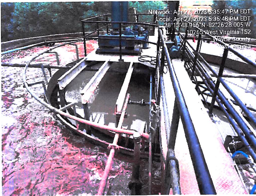
Pollutant in the Town of Wayne's wastewater treatment plant.
