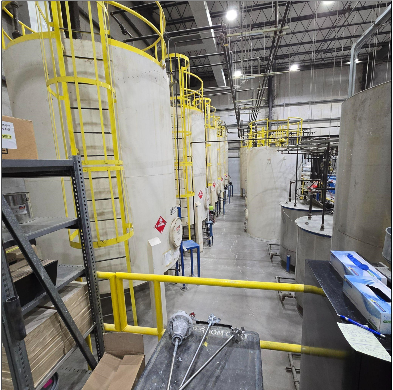
April 28, 2025 – Aboveground storage tanks (ASTs) in the secondary containment area of the pump room.
