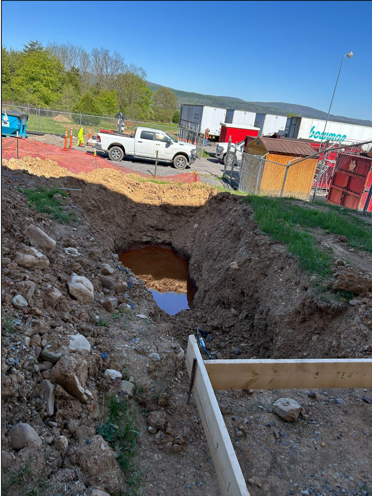
April 28, 2025 – Excavated area where a chemical odor was noticed in the groundwater.
