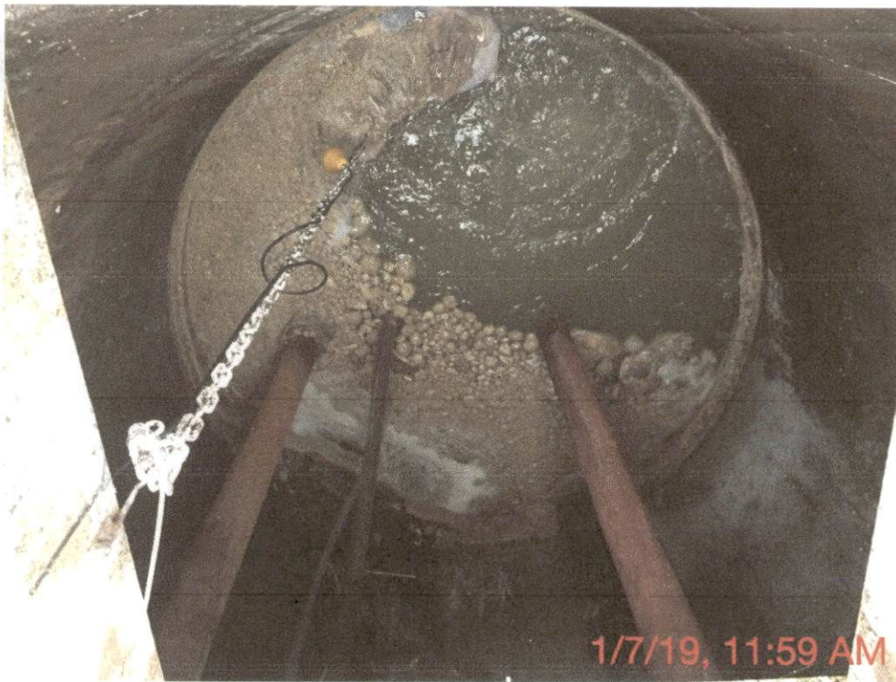
Maddex lift station well with grease
