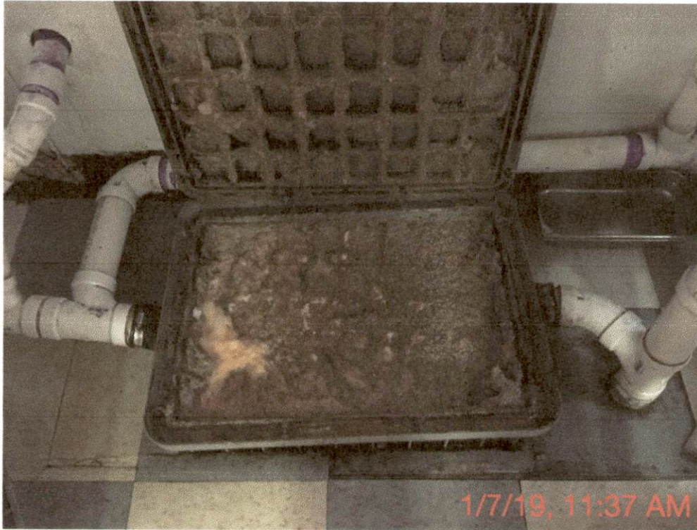
Blue Moon restaurant grease trap, full of grease
